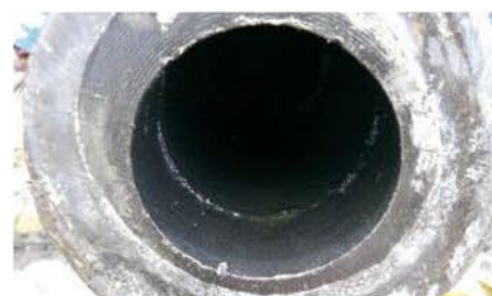
Thermoflow ® treated pipeline
